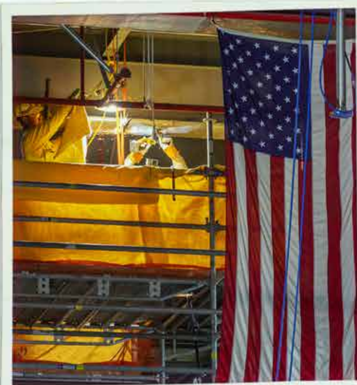
Ironworkers prep structural steel for pipe supports installation in the Main Process Building.
